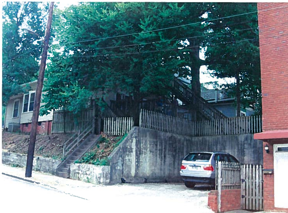
Fig.1 - Overall conditions of existing wood deck, parking area and access to second floor deck.
